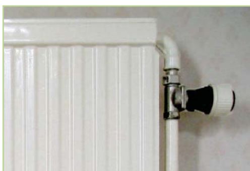
Radiator valve at a height of 800 mm
