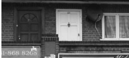
Inappropriate small scale alterations to residential flats
