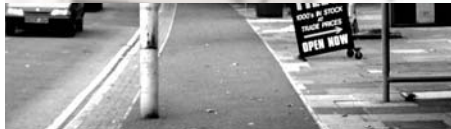
Patchy pavement surfaces
